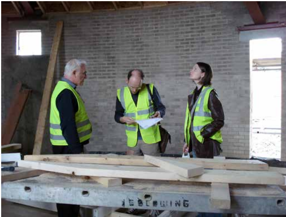
Artists checking their studios on site during the construction of Manor Oaks Studios. Photo: Yorkshire Artspace.
