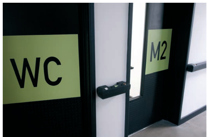
Example of door signage and helping band
